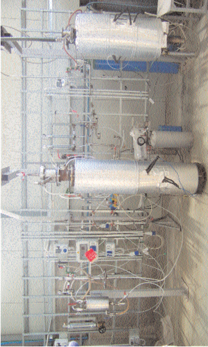
Fig. 3. Laboratory scale fluidized bed reactors in the area of Le Calorie S.p.A. that is available for the experimental activity of the Department of Environmental Sciences of Second University of Naples.
